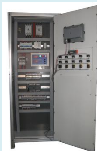
Control cabinet internal view
