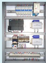
Control cabinet internal view
