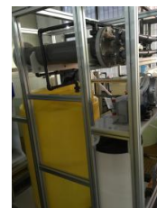
Alkali tank + alkali recover system
