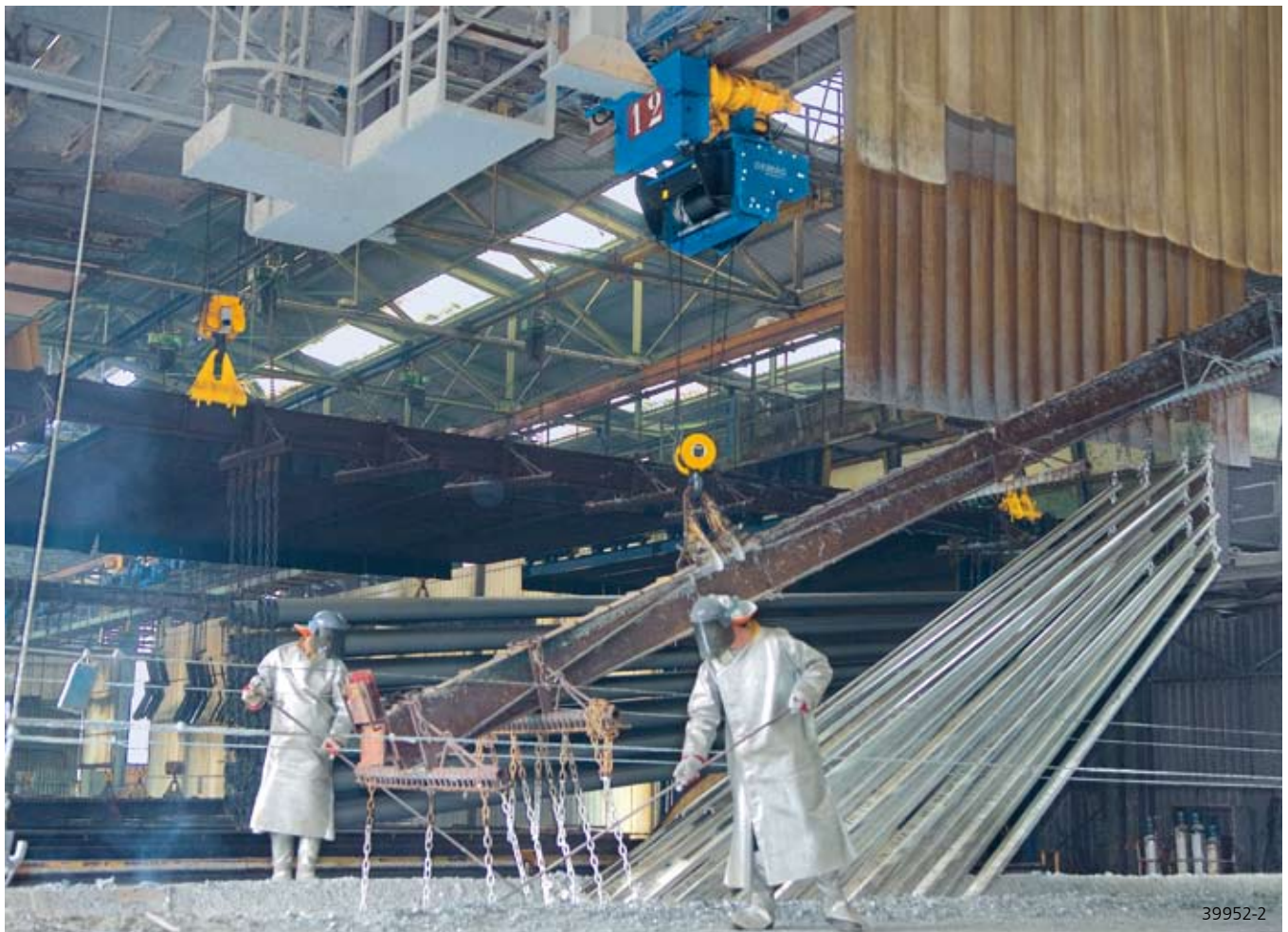
Demag FDR foot hoists travelling on a semi-automatic circuit in a galvanising plant.
